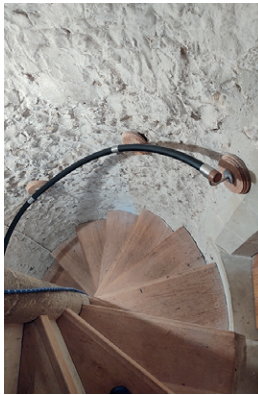
Old stone steps, capped with wooden treads, providing access to the Bell Chamber and Tower
